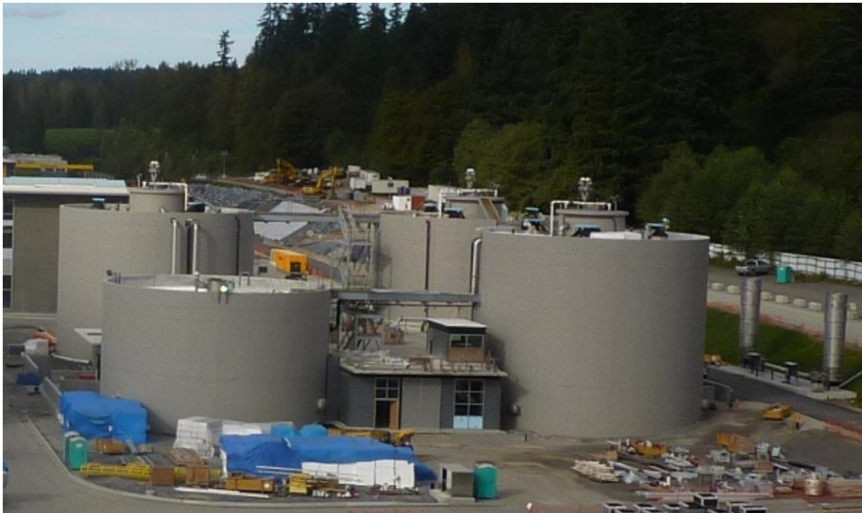
Figure 4-3. Silo-style digesters (taller) and sludge storage tank (shorter) under construction at the Brightwater WWTP, Woodinville, Washington
