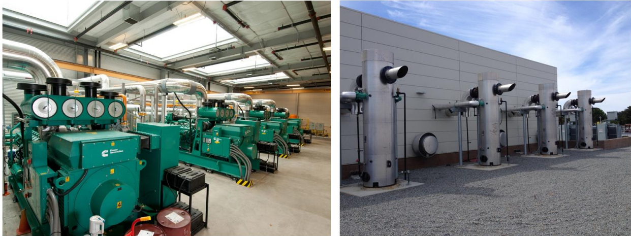
Figure 3-9. CHP facility with (4) 1.1-megawatt IC engines and post-combustion treatment
