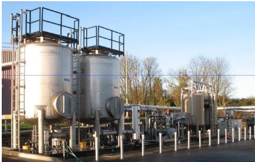
Figure 4-7. Digester gas treatment system, Columbia Boulevard WWTP
