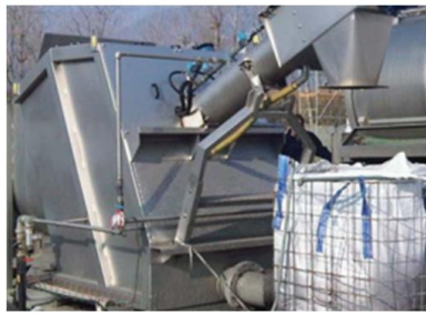
FOG Receiving Screen pilot at HRSD wastewater plant
