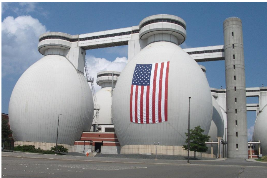
Figure 3-6. Egg-shaped digesters at the Deer Island Treatment Plant, Boston, MA
