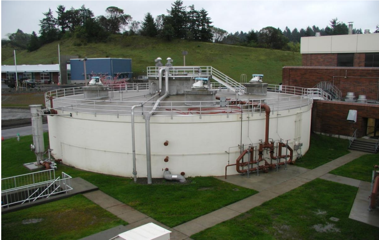
Figure 4-4. Short-cylinder (a.k.a. pancake) style digester at the Chambers Creek WWTP, University Place, Washington
