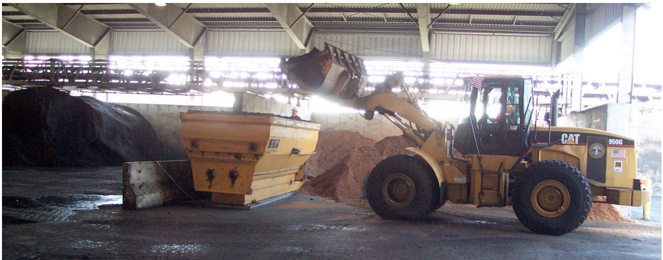
Composting solids at Southbridge, MA.
